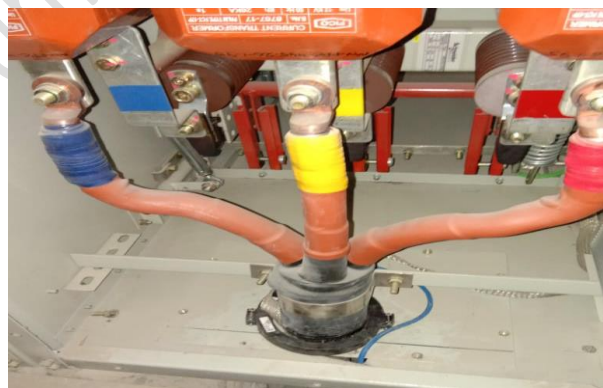
Figure 18 - Cable Termination of VCB
