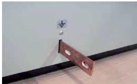
Figure 17 - Earthing Terminal on VCB Panel
